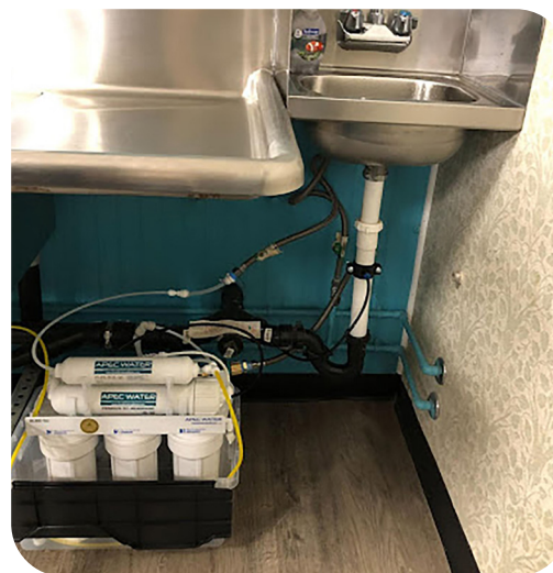
Point-of-use water filtration system designed and installed by AW4A engineers in Florence, Arizona
